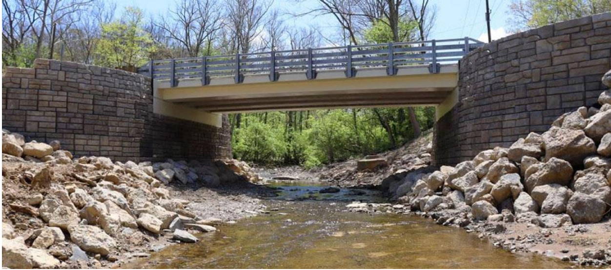
Figure 13. Large-block bridge abutments in Hamilton County, OH that resulted in $40,000 cost savings (Redi-Rock 2020)
