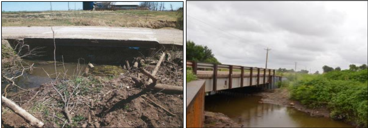
Figure 20. Before and after pictures of the GRS Bridge No. 3 in Kay County (Photographs Courtesy of Mr. Tom Simpson, PE)
