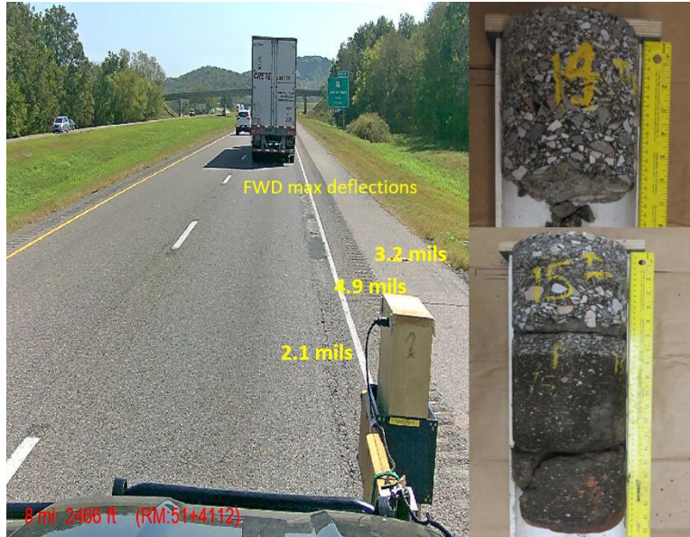
Figure 2.3 Lane and shoulder segments of I-35 near Mile Post 51.5 and extracted cores
