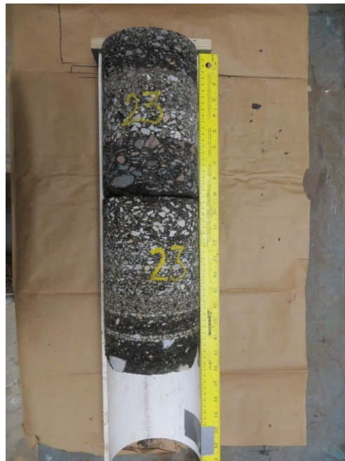
Figure A.14 Core #23 on SH-7
