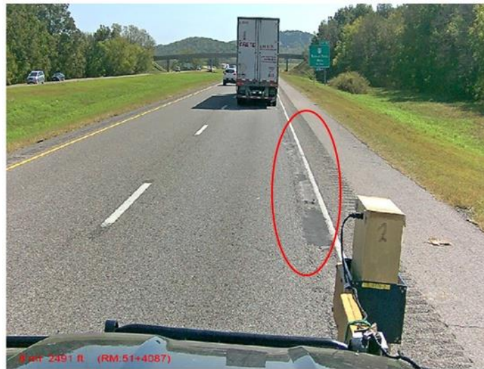
Figure 1.1 Longitudinal edge cracking observed on I-35
