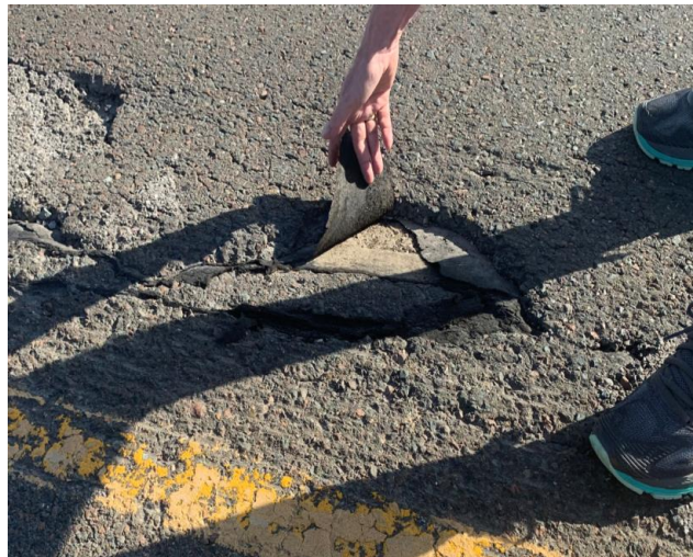
Figure 1.4 Photographic view of delaminated fabric layer on SH-7
