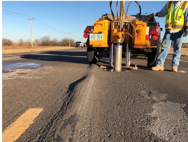
Figure 1.3 Photographic view of rut observed on SH-7
