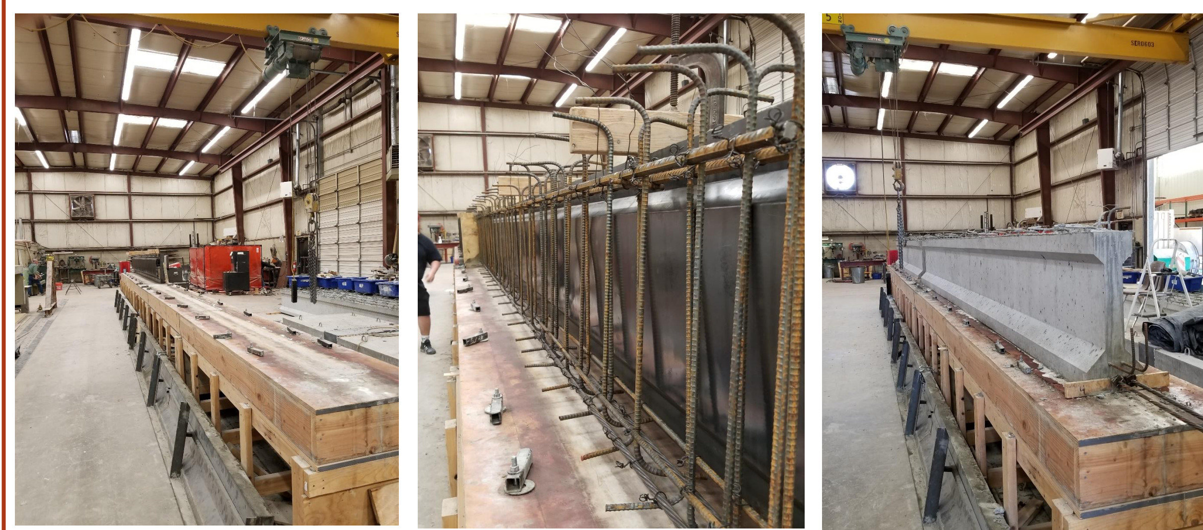
Preparing the Prestressing Bed for Formwork at Fears Lab Prestressing Strand/Shear Reinforcement Placement Detensioning the Strands after 24 Hours to Complete the Beam Construction
