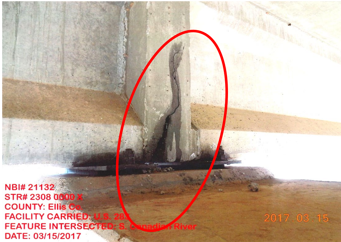
Typical cracking in continuity connection on U.S. 283 over S. Canadian River (Photo courtesy of Walt Peters)
