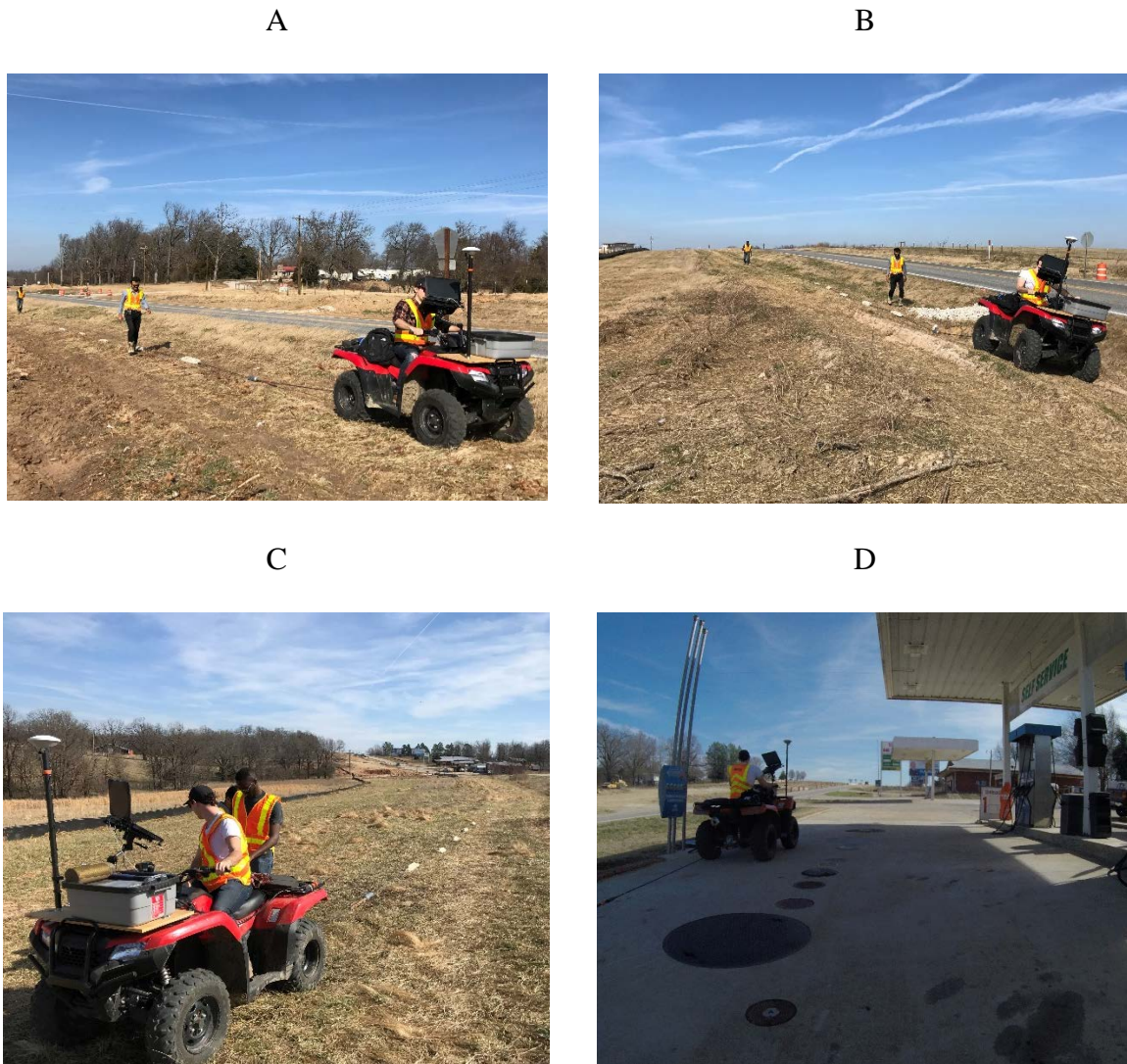
Figure 3-10. Along the Alpena Highway alignment OhmMapper towed at; A) STA 403+00 right side of highway, B) STA 451+00 passing over a buried utility crossing the highway on the right side, C) STA 484+00 left side of the highway, D) STA 491+00 passing through a gas station on the right side of the highway.
