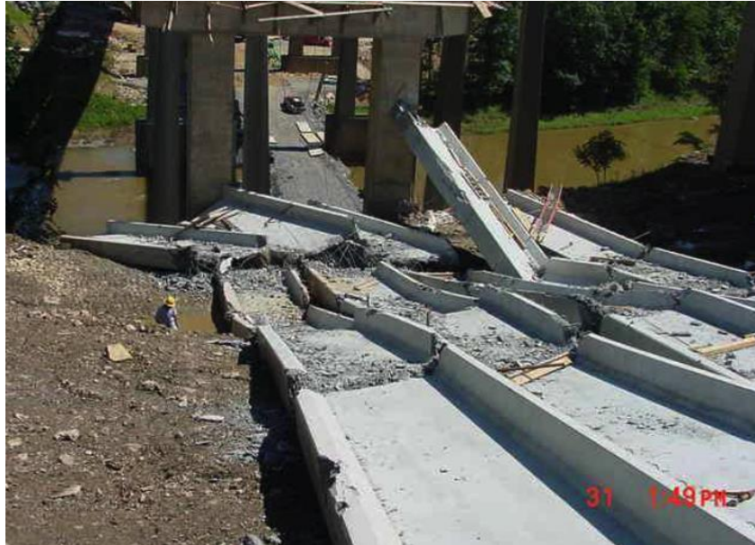
Figure 1.2 - Collapse of I-80 girders in Pennsylvania (Lee, 2010)
