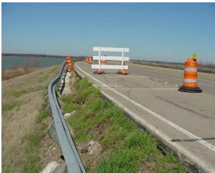
Figure 23. Slope Failure on Lake Ridge Parkway (Gregory 2006)
