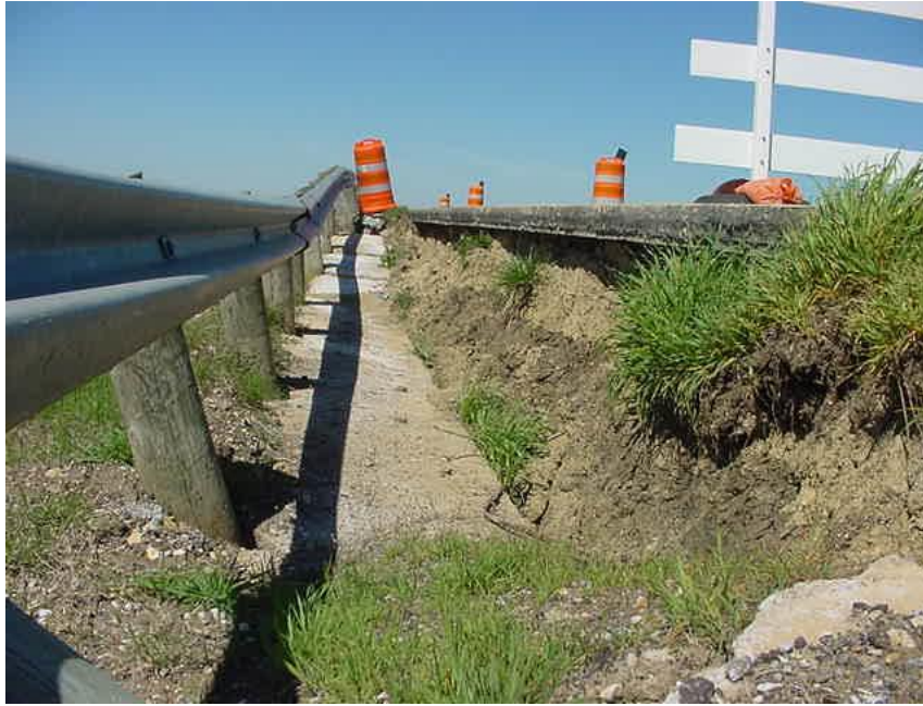
Figure 24. Slope Failure at Roadway Edge - Lake Ridge Parkway (Gregory 2006)
