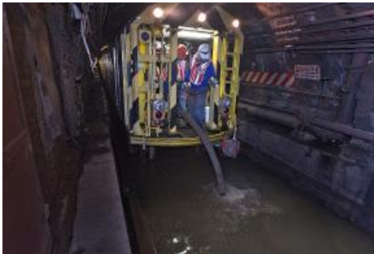
Figure 25. Flooding in a Subway Tunnel in New York City after Hurricane Sandy [53]
