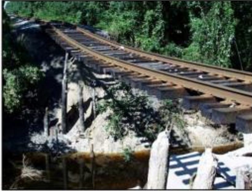
Figure 26. Railroad Bridge Washed Out by Hurricane Flooding [42]
