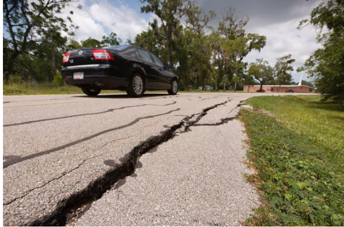
Figure 20. Cracks in a Pavement Due to Drought in Texas [36]
